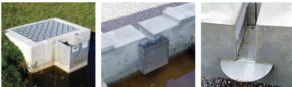
Figure 28.27 Examples of debris guards over low-flow outlet control structures (courtesy Robert Bray Associates)
