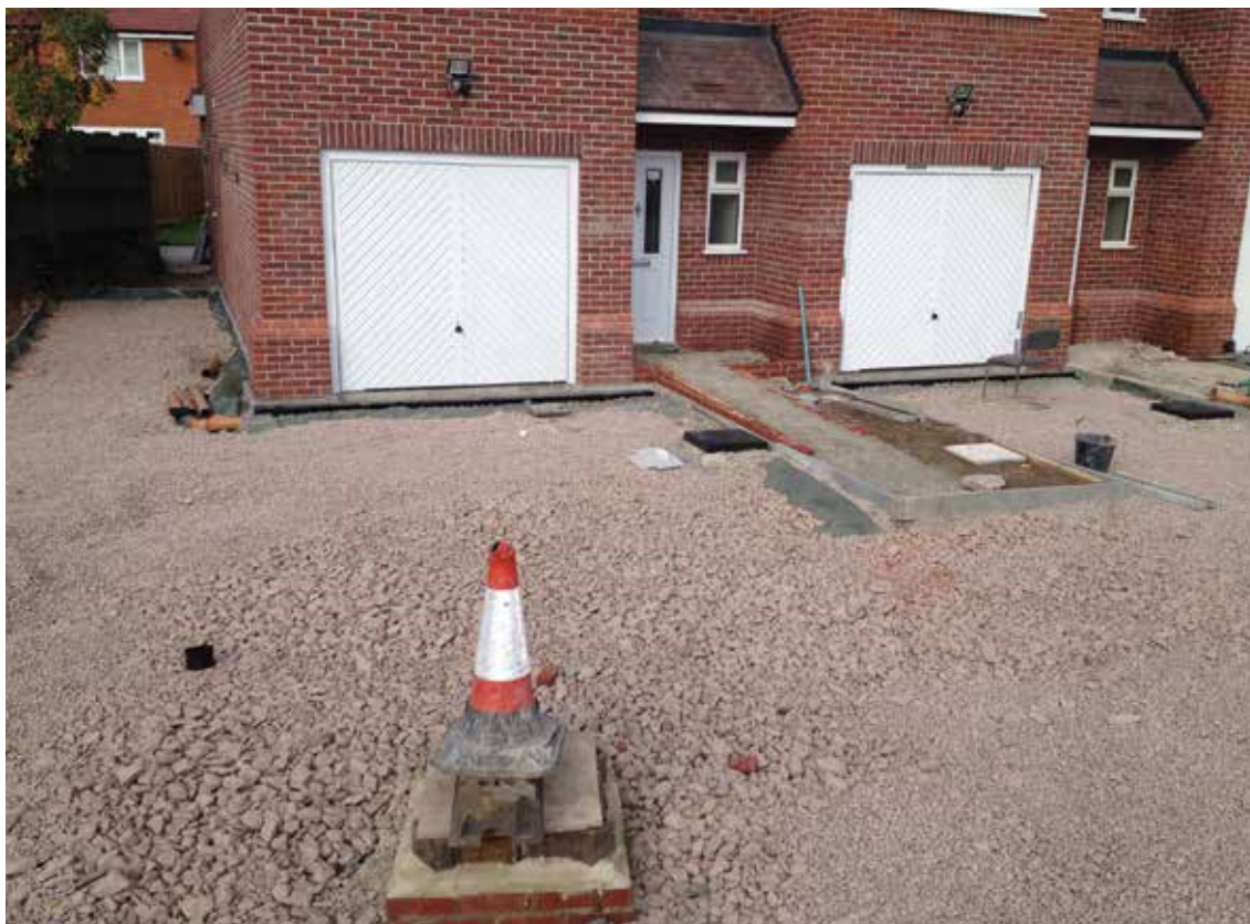
Figure 31.3 Concrete block permeable paving being constructed at the end of the project (courtesy EPG Limited)
