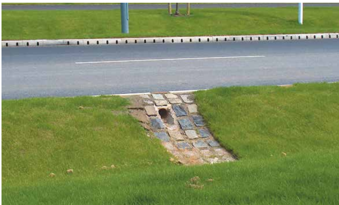
Figure 28.7 Kerb collection system being used to drain a carriageway in conjunction with a swale (courtesy ACO Limited)
