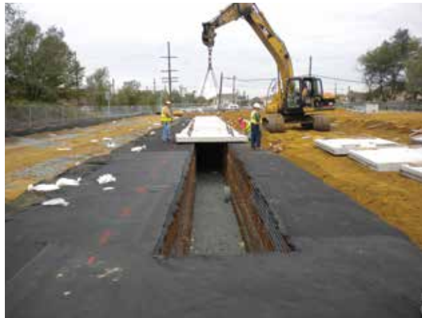
Figure 21.15 Hybrid tank of reinforced earth and concrete roof panels (courtesy Stormwater Management)
