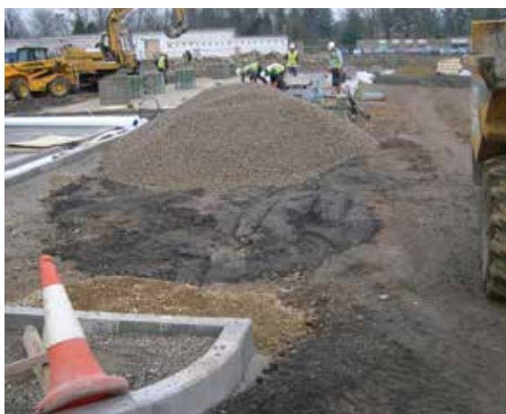
Figure 31.1 Inadvertent compaction of subgrade below pervious surface construction intended to infiltrate water to ground. Compaction will reduce the infiltration rate (courtesy EPG Limited)
