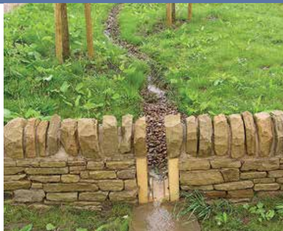
Figure 6.2 Conveyance component (courtesy Sheffield City Council)
