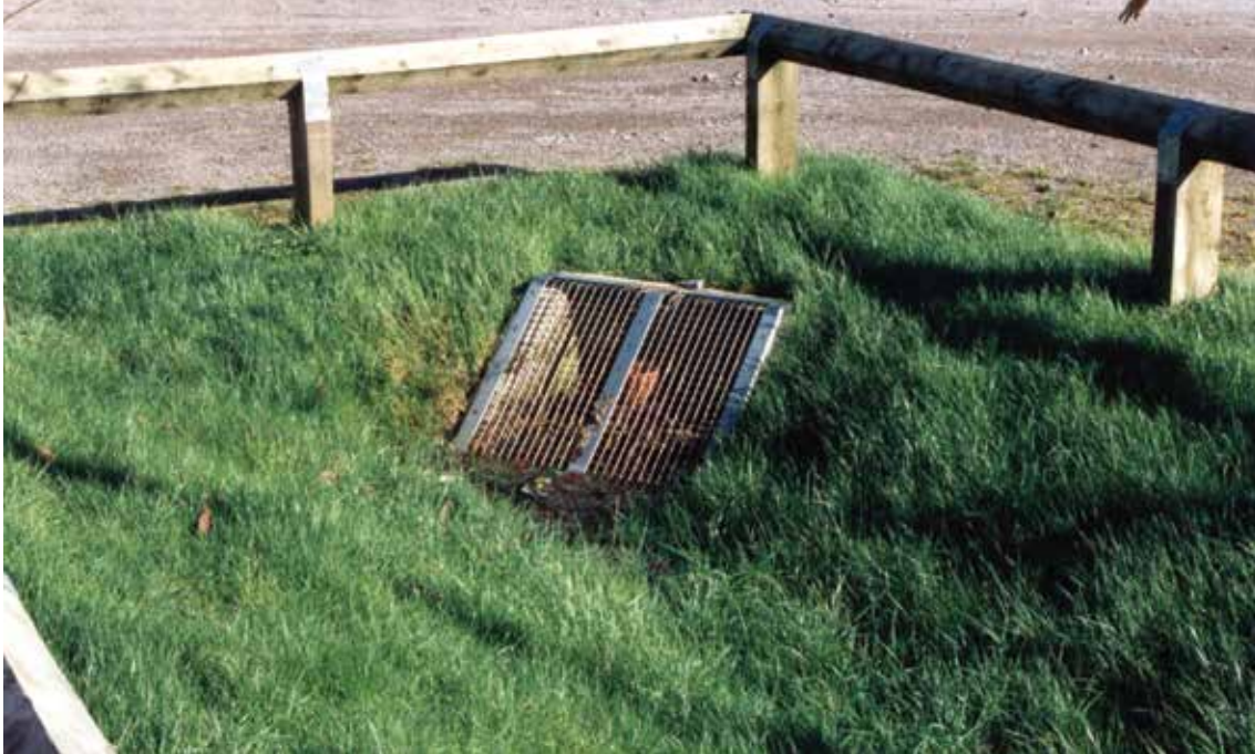
Figure 28.15 Example of screened orifice outfall with T-piece structure (courtesy Robert Bray Associates)
