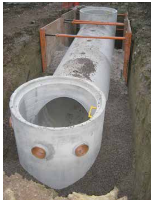
Figure 21.9 Direct access chamber into concrete pipe (courtesy British Precast)
