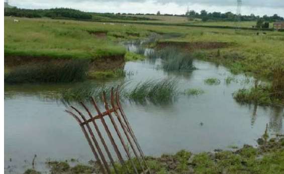
B: Active reach with bank erosion (JBA, 2013)
